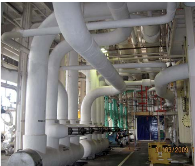
Turbine Hall Pipework (Lagged)
