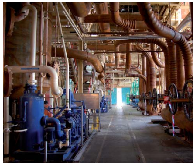
Turbine Hall Pipework (Stripped)
