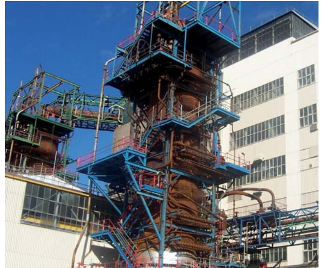
Heat Exchanger (Stripped)
