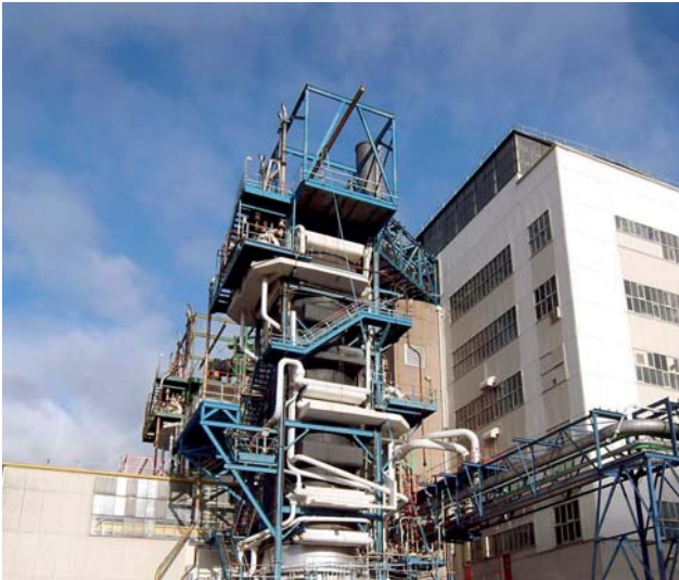
Heat Exchanger (Lagged)
